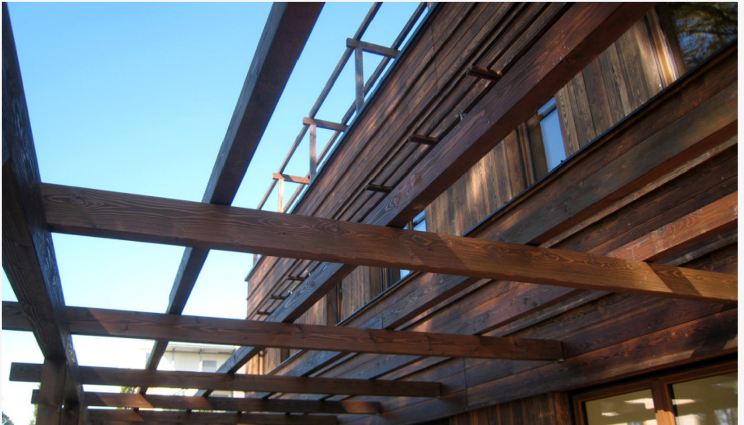
City of Wood was a project for prefabricated social housing in Bad Aibling, Germany, where terraced houses with wooden facades are merged with surrounding nature. Photos: MTP
